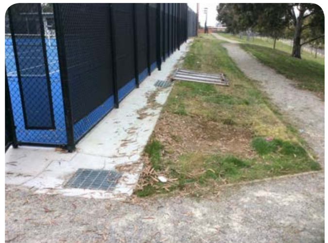
Concrete spoon drain with corner junction pit and intermediate pit for added capacity. Note: debris in the form of grass clippings requires continual maintenance to keep the system functioning as intended.
