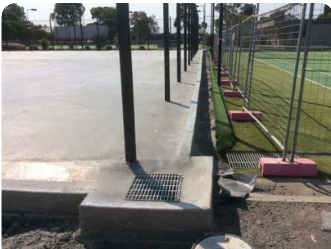
Concrete spoon drain and stormwater grated pit cover. This is located at the lowest corner.
