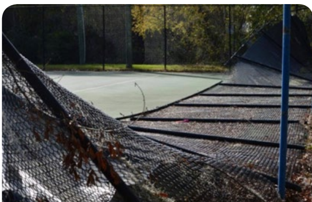
Example of a collapsed fence fitted with windbreak material caused by inadequate design.
