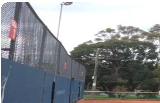
Example of installation of windbreak material on a non-strengthened fence that has resulted in structural failure.
