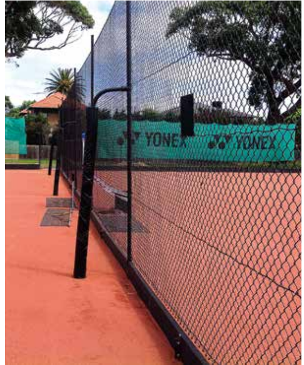
Image 3.2.6 & 3.2.7 Incorrect backstay placement
