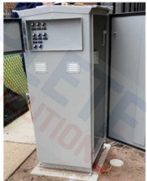
CAAMS Enclosures housed in a small size freestanding switchboard enclosure with custom key switches located on the side of the switch board enclosure*
