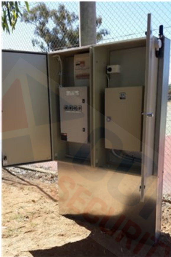
CAAMS and LCP Enclosures housed in a medium size freestanding switchboard enclosure
